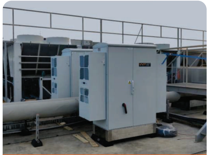
Carrier 50 ton Air-Cooled Chillers - Crane Currency
