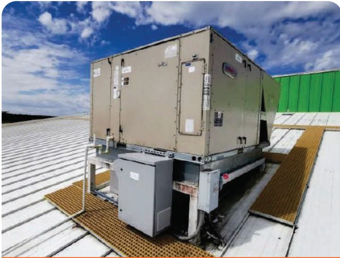
Lennox RTU - Walmart owned Supermarket
