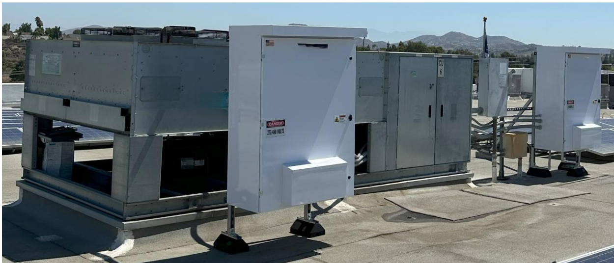
Figure 25: Site 2 CU6E and CU6W compressors with the ET.
