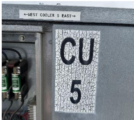
Figure 17: Site 2 CU5 condensing unit nameplate with CU5E and CU5W.
