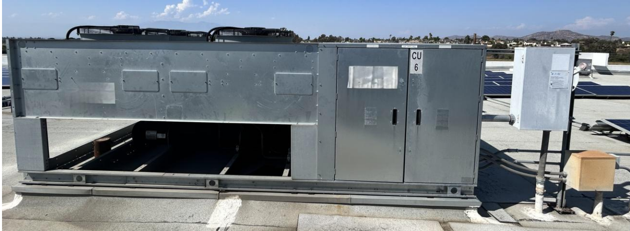
Figure 18: Site 2 CU6 condensing unit with CU6E and CU6W.
