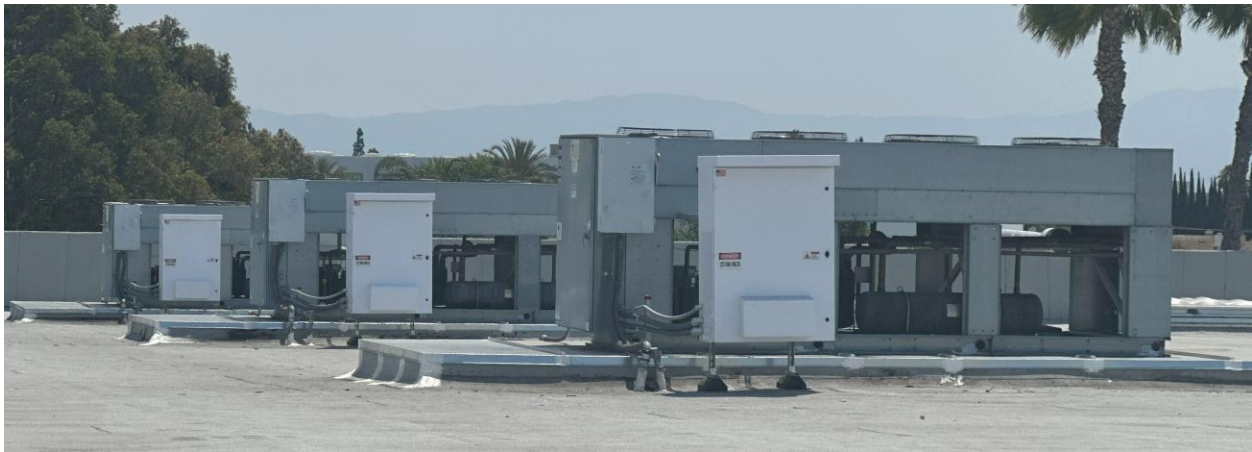
Figure 15: CU4, CU5, and CU6 condensing units with the ET.
