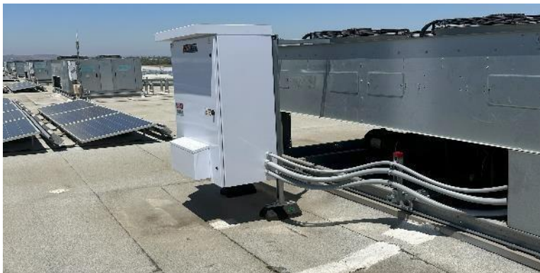
Figure 23: CU5E compressor with the ET.
