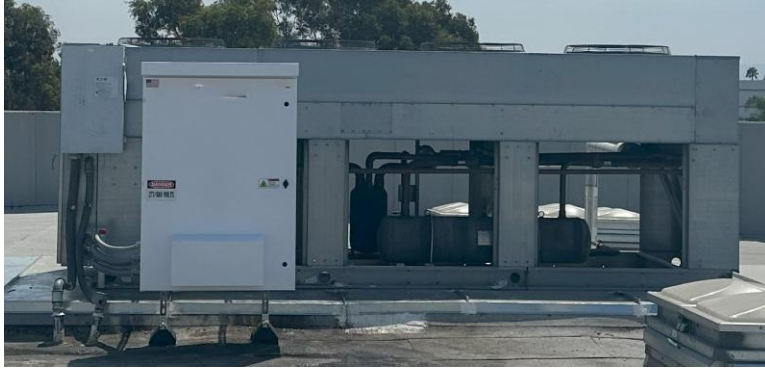
Figure 14: CU3 condensing unit with the ET.
