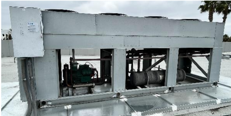
Figure 6: CU3 condensing unit.
