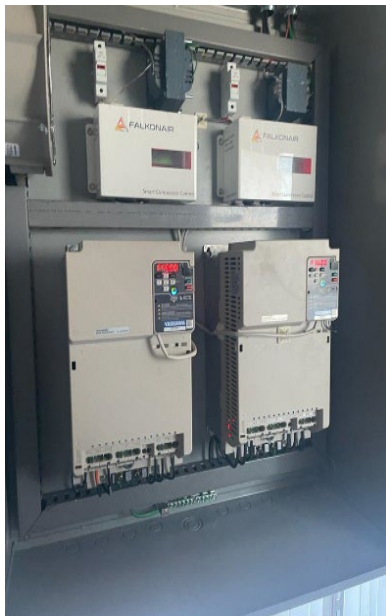
Yaskawa VFD's with SCC's
