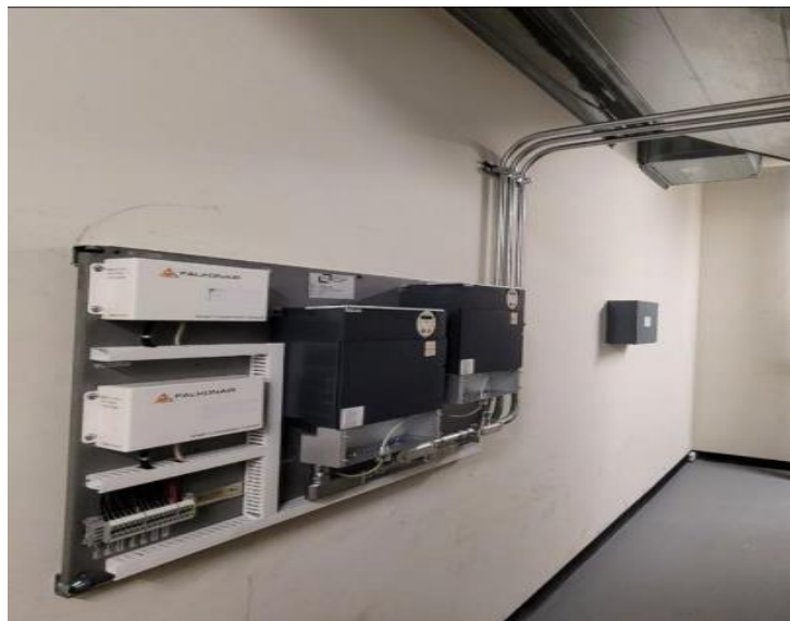
The Schneider Dual VFD Panel
